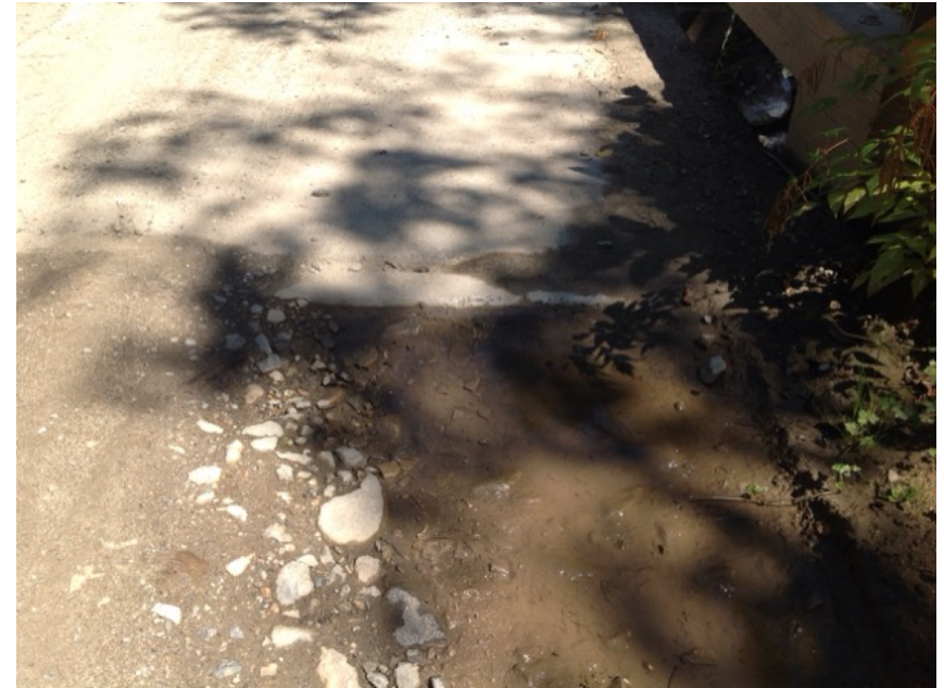
potholes at approaches
